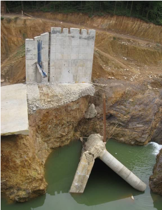
The breached dam which released an estimated 28 million tonnes of water (and the turtle) over a two-day period. Amazing that the turtle survived. this escape...
